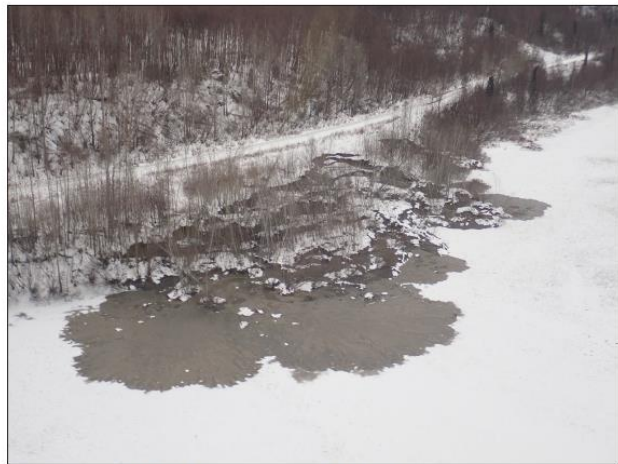
Complex earthflow slumping along Alaska Railroad overlooking tidal flats along Knik Arm near Mirror Lake.
